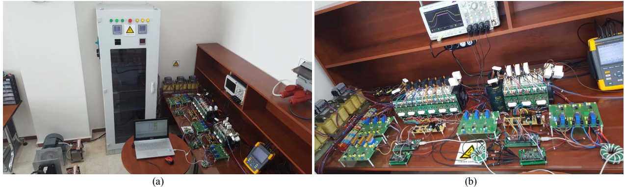
Figure 7. Experimental setup (a) the complete hardware (b) only power converters.
