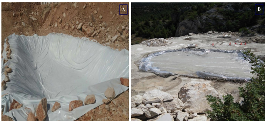
Fig. 2 a, b Construction and use of clarification tanks
