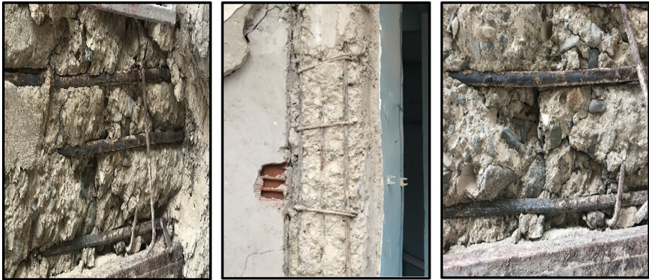
Fig. 1 Damaged RC columns in old buildings, smooth bar and low transverse reinforcement content (Caglar et al. 2022)
