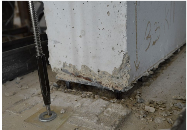
Fig. 12 Crack at base level in specimen NCSW2
